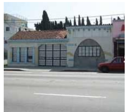
Concrete block is not a material that is original to this Spanish Colonial building.
